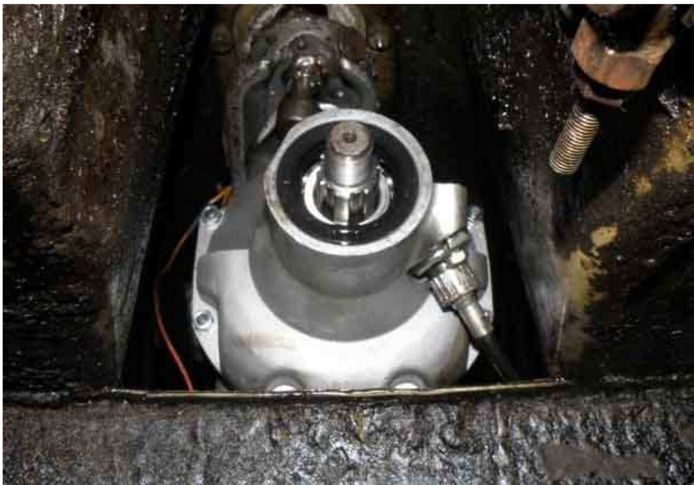
The 'ice pick', and the large socket that was used to drift the new seal into position
